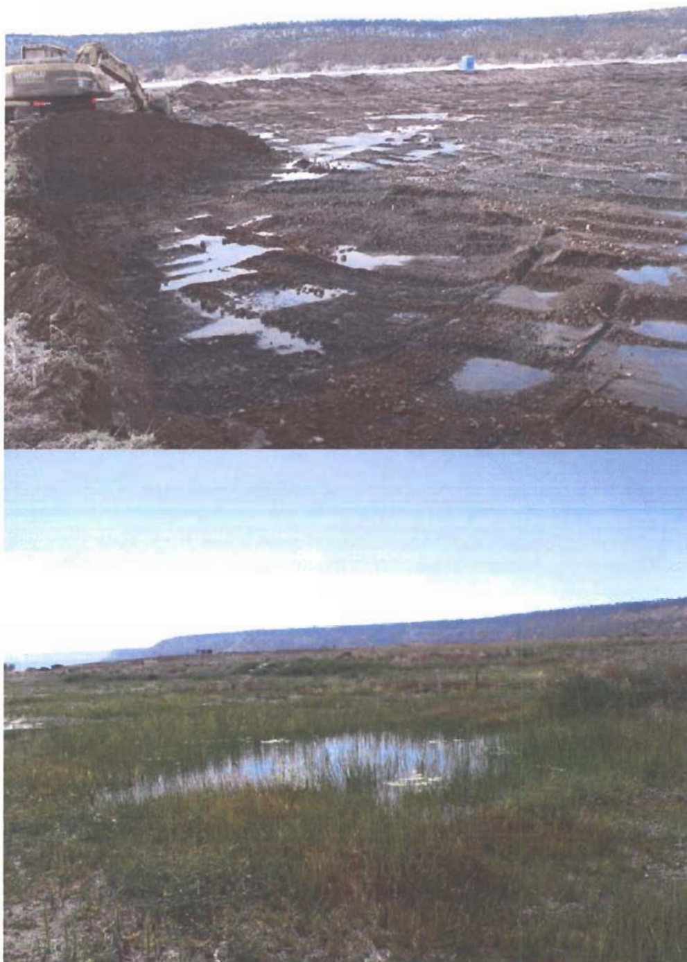
Figure 5-6. Constructed wetland at the City of Prineville wastewater treatment facility during excavation (Feb. 2005), and at the end of the first growing season (Sep. 2005)
